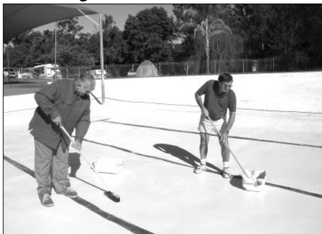
Paint job. Peter Ryan, manager Caravan park & pool (left), and workman Walter putting 440 litres of 'Olympic blue' paint on Nimbin pool.
